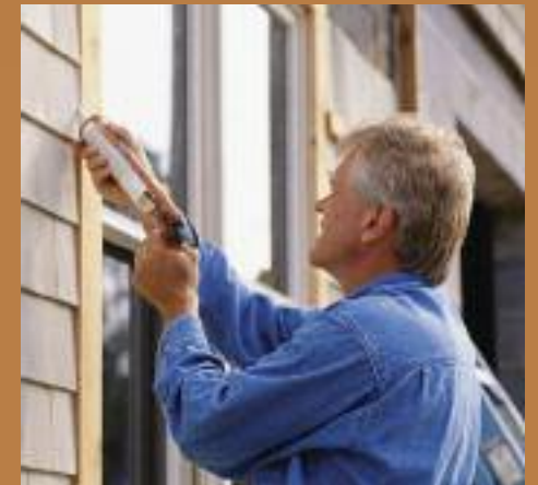
Most energy efficiency experts will stress that a couple of tubes of caulk go a long way toward providing big energy savings in the home.
