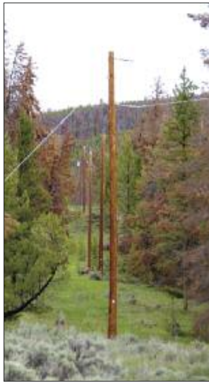
Many of Mountain Parks Electric's distribution lines are threatened by dead and dying lodgepole pine trees that can fall on conductor, knock out power and possibly cause a major wildfire. Photo by Les Shankland of Mountain Parks Electric.
