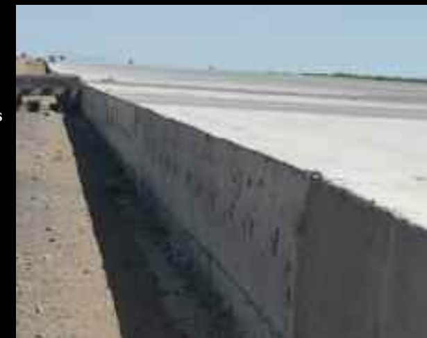
Construction on the two-mile runway was completed in August. A 45-ton paving machine formed the runway in concrete strips, each 30 feet wide and 14 inches thick.
