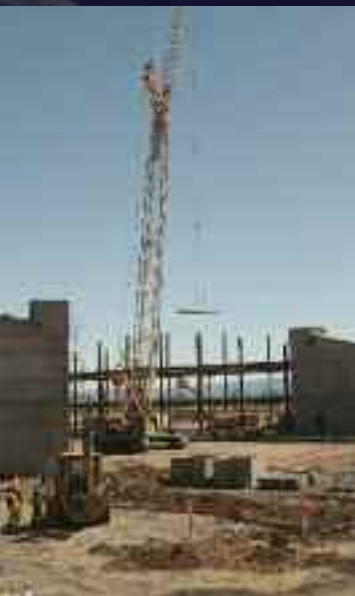
A 47,000 square-foot hangar will house Spaceport America tenants, including Virgin Galactic. The hangar was designed to achieve LEED Gold standards, including the installation of Earth Tubes, solar thermal panels and under-floor radiant cooling and heating.
